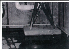
Wet basement before EOP application
